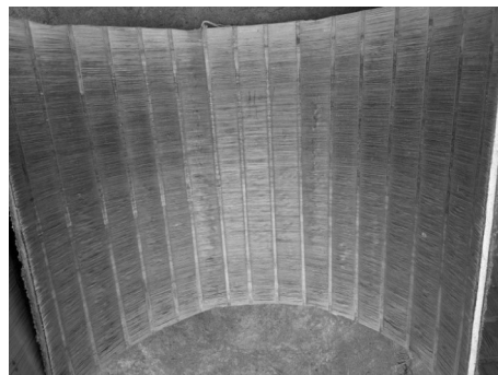
图8 B相电抗器第11包封 Fig. 8 The 11th envelope of reactor of phase B
