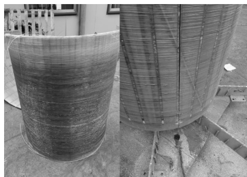
图9 B相电抗器第12包封 Fig. 9 The 12th envelope of reactor of phase B
