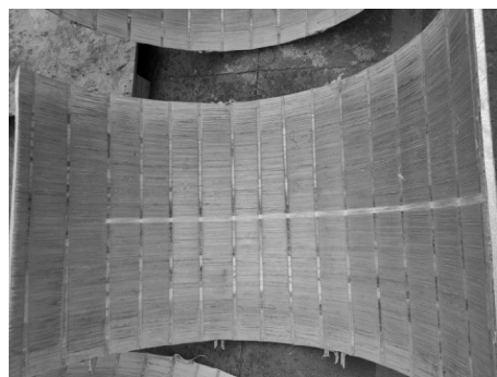
图7 B相电抗器第10包封 Fig. 7 The 10th envelope of reactor of phase B
