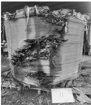
图4 C相电抗器第11包封 Fig. 4 The 11th envelope of reactor of phase C
