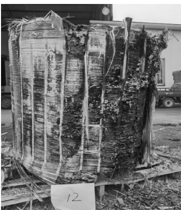
图5 C相电抗器第12包封 Fig. 5 The 12th envelope of reactor of phase C
