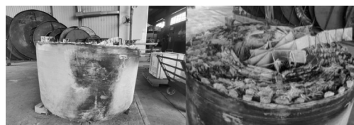
图1 C相电抗器烧毁情况 Fig. 1 Burnt-out condition of reactor of phase C
